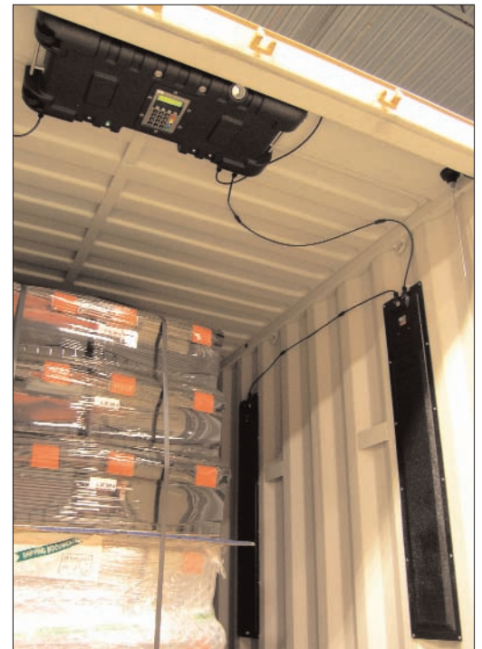
The SMART Container’s control unit (shown attached to the container’s ceiling) works in conjunction with the Blackbird Wing, which functions as an RFID portal.
