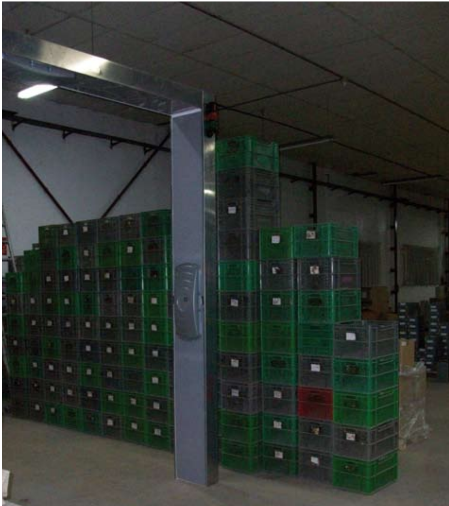
RFID portal located between the warehouse and quality control
